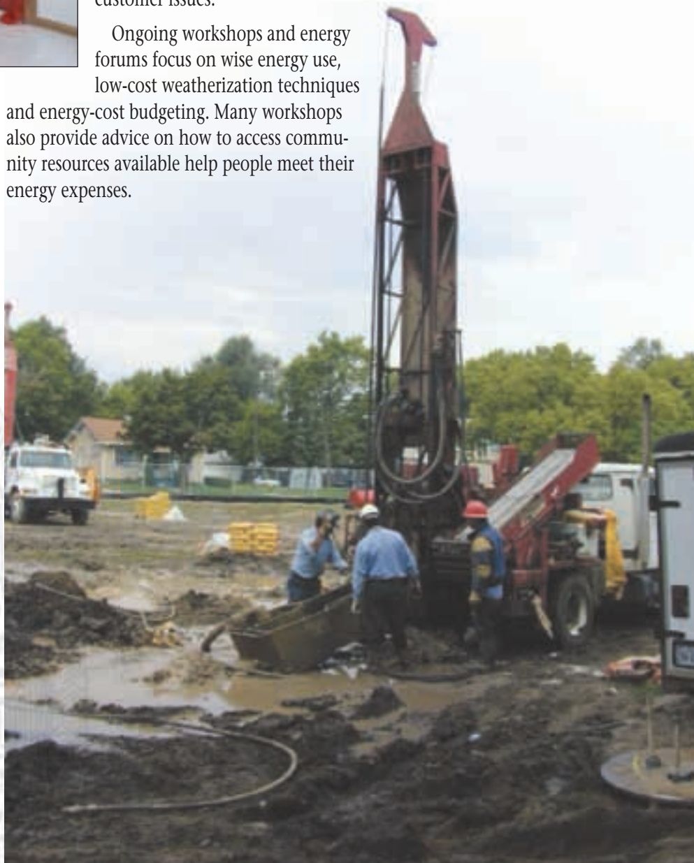
LES oversees the installation of a geothermal well at Clinton Elementary School.
