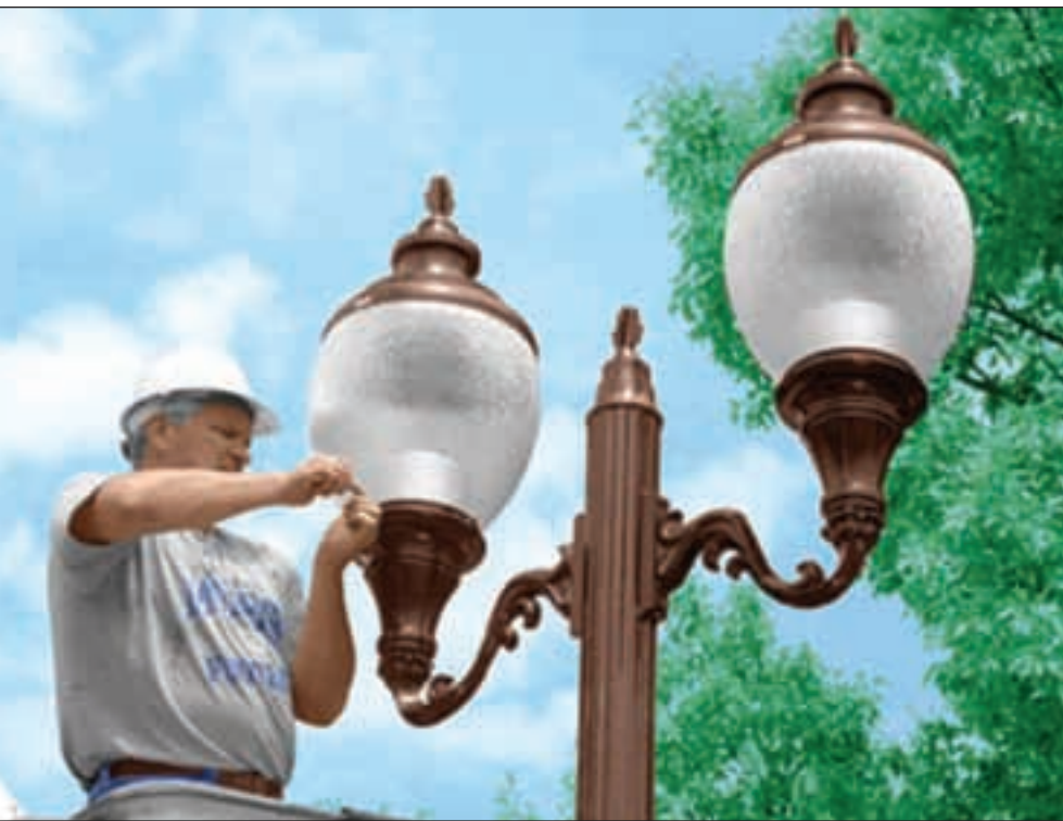
The city of Tecumseh used an Energy Efficiency and Conservation Block Grant to upgrade its city streetlights.
